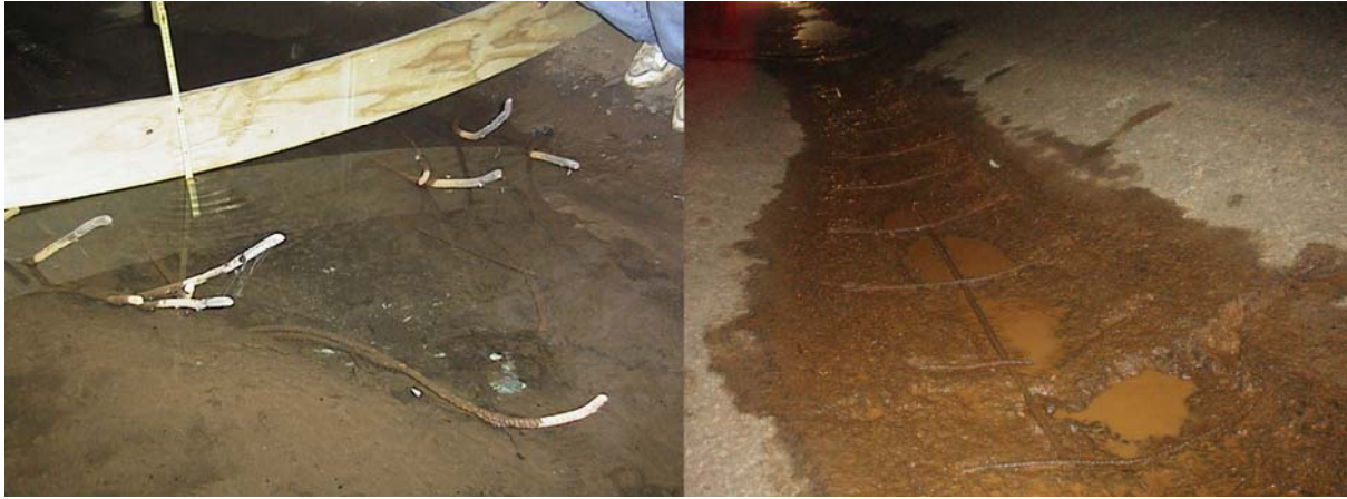
Figure 4-Erosion along tunnels invert zones
